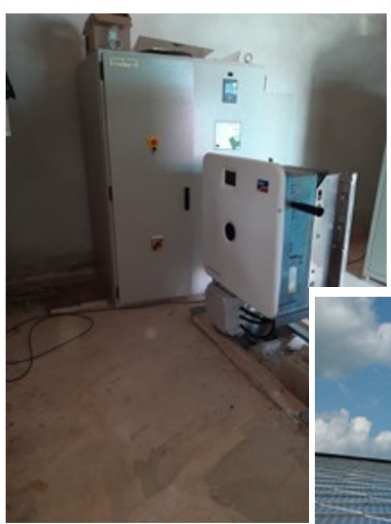
New Inverter - SMA
