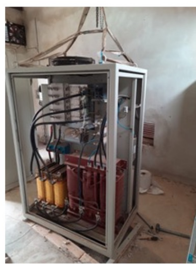
Old Inverter - GPtech
